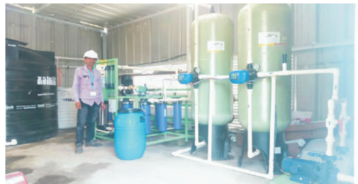
5000 LPH RO Plant
