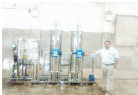
2000 LPH Fully Automatic SS RO Plant
