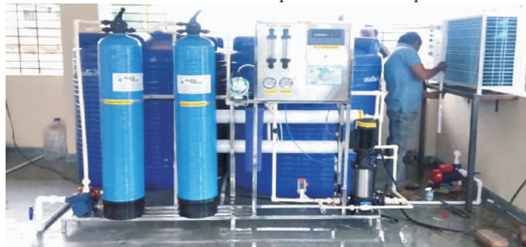
500 LPH RO Plant
