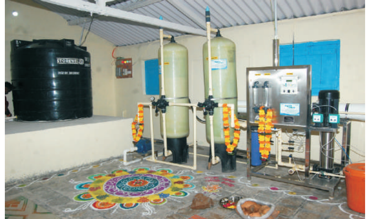
4000 LPH RO Plant
